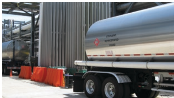
Interim gas flow outages utilizing 2-80 K vaporizers
