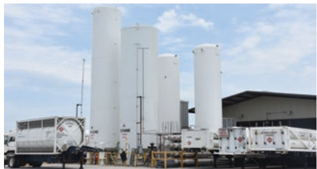
Hydrocarbon Storage Facility
