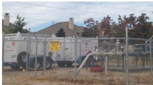
Residential utility pipeline support
