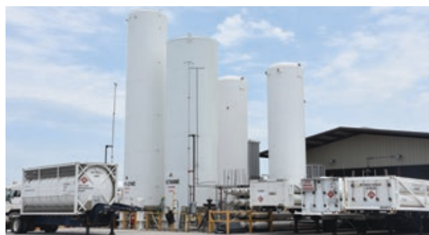
Hydrocarbon Storage Facility
