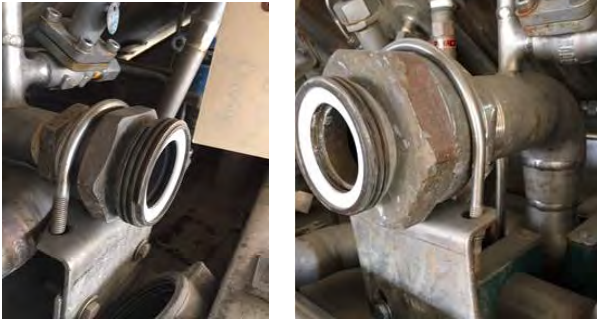
3 1/4 ACME TRAILER TANK CONNECTION
