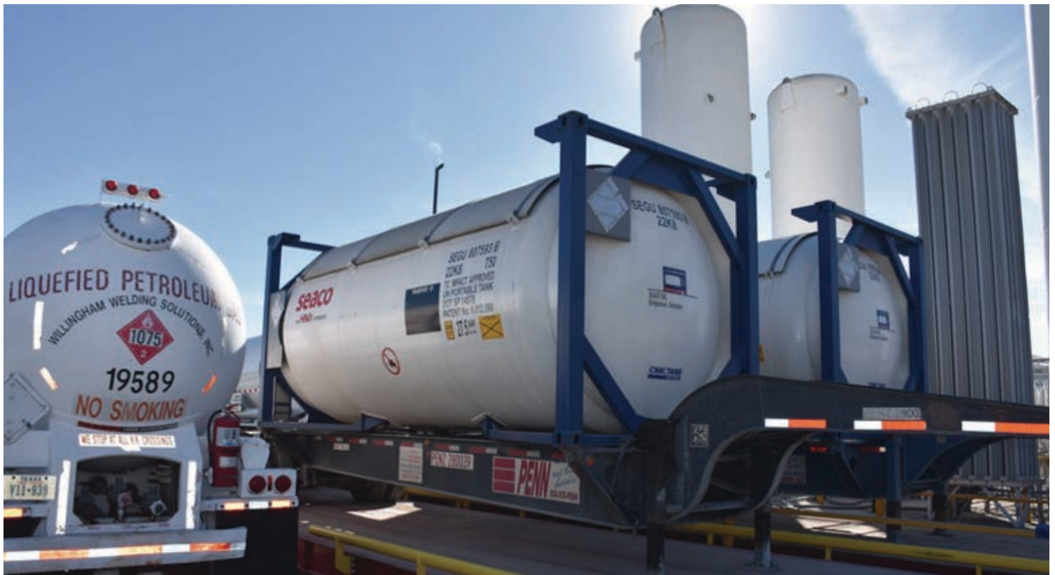
Source: Gas Innovations
